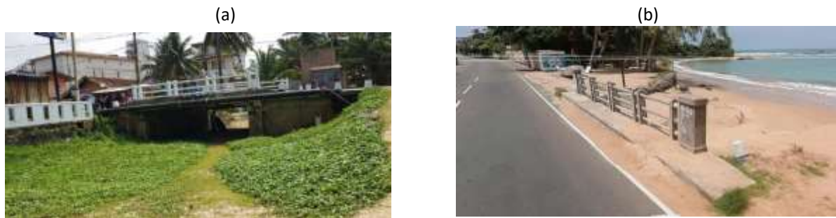
Figure 10: Outlets of Tuduwegoda canal (a) Mawakada canal (b) are filled with sand
