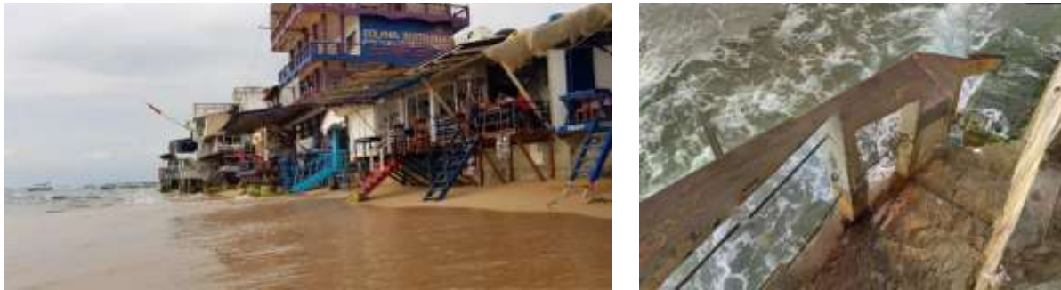
Figure 7: Coastal erosion in the north section of the Hikkaduwa beach Source: Field observations, 2022
